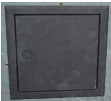
Access hatch in a sanitary plumbing stack
