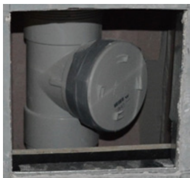
Inspection opening in a sanitary plumbing stack
